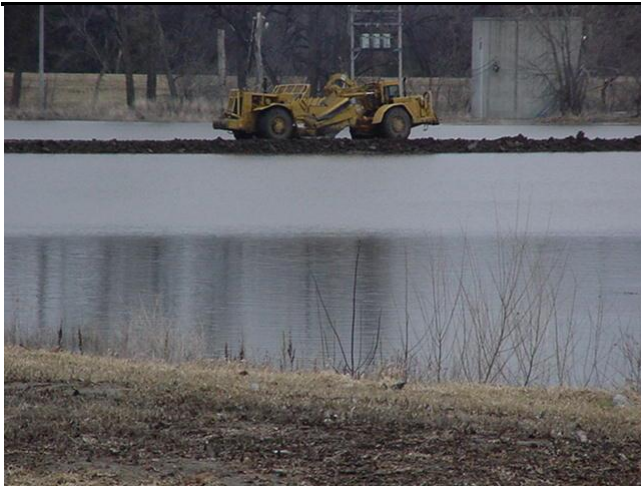
A 627 hauls across a make shift road out in to the river, we lost this pit at 42ft.
