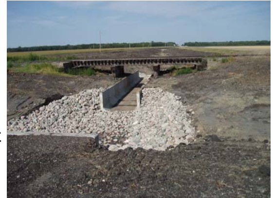
Box Culvert under the R.R. Tracks on the Ditch No. 46 job. Nice job guys!
