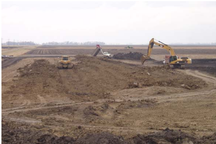
(above) The guys put the finishing touches on the Lime Landfill Levees at Drayton Crystal Sugar Plant
